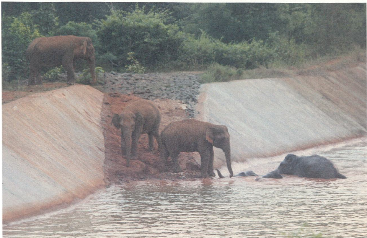
Figure 3.3.14: Ramps/exits similar to these built on canals, to facilitate escape of wild animals in the event of approaching trains in the walled sections Kalabil (Ch. 15/2 – 15/6), and that near Gamani Ban Gaon (Ch. 22/0 – 22/4) should be provided [Picture courtesy: Jagyandatt Pati]
