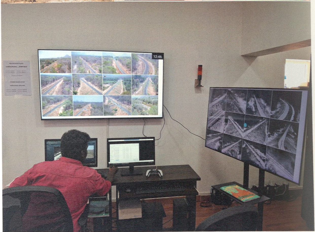
Figure 3.9.4: AI-based elephant monitoring and alert system on railway tracks in Madukkarai Forest Range. Top left- cameras are installed on towers close to the railway line; Top right- the control room; Bottom- Continuous monitoring in action.
