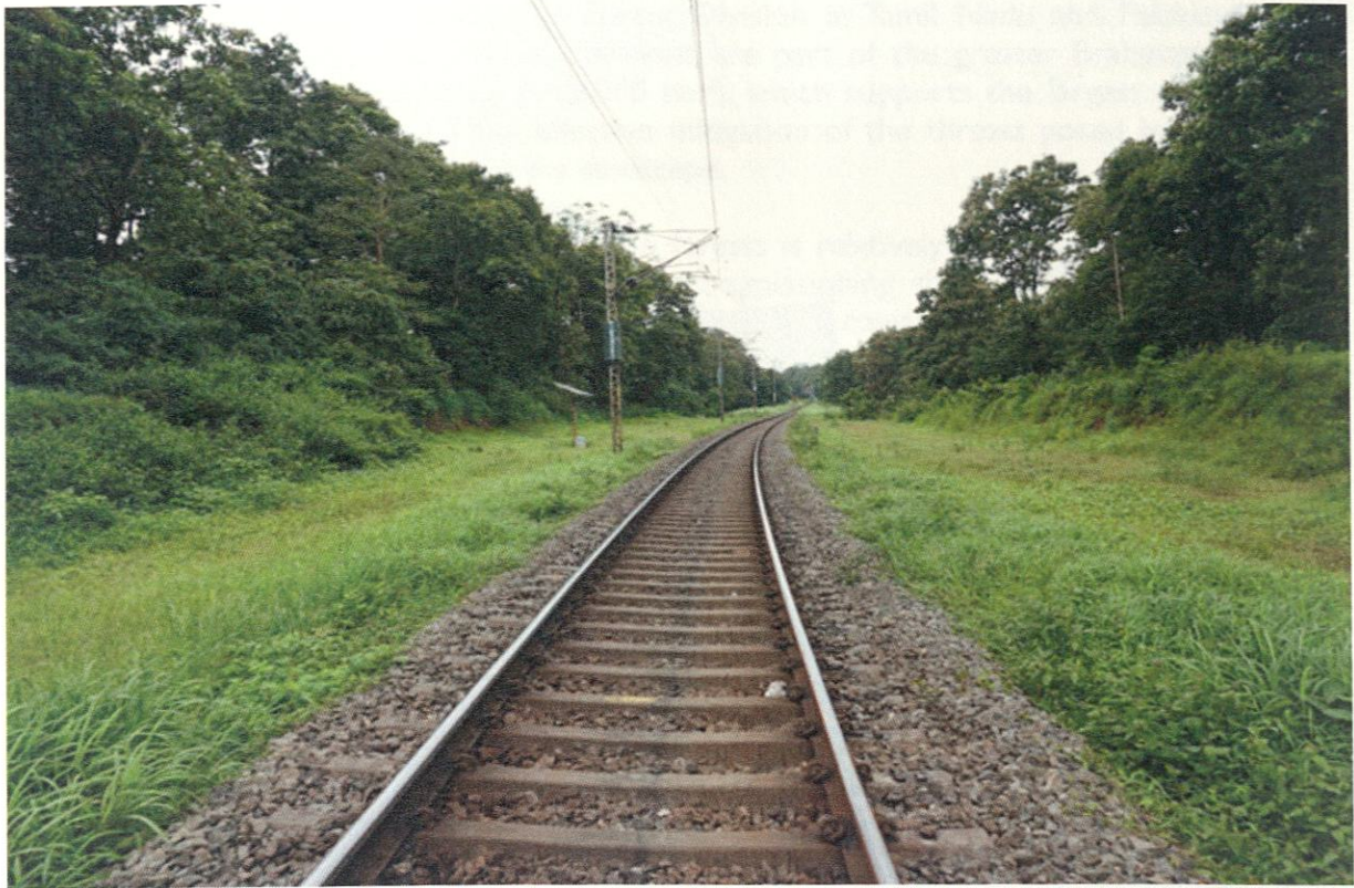
Clearance of vegetation (vista clearance) along the Railway line for about 10 meters as seen in Track B of the Kanjikode (KJKD) – Walayar (WRA) section
