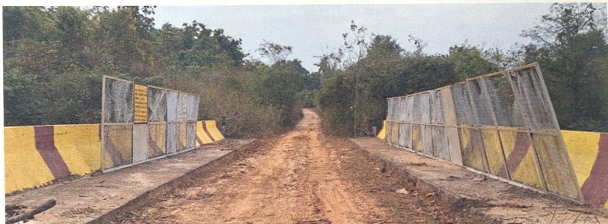
Figure 3.4.4: Existing mitigation measures need modification like barricading from the side of the overpass along the along railway track and placement of light/sound barriers
