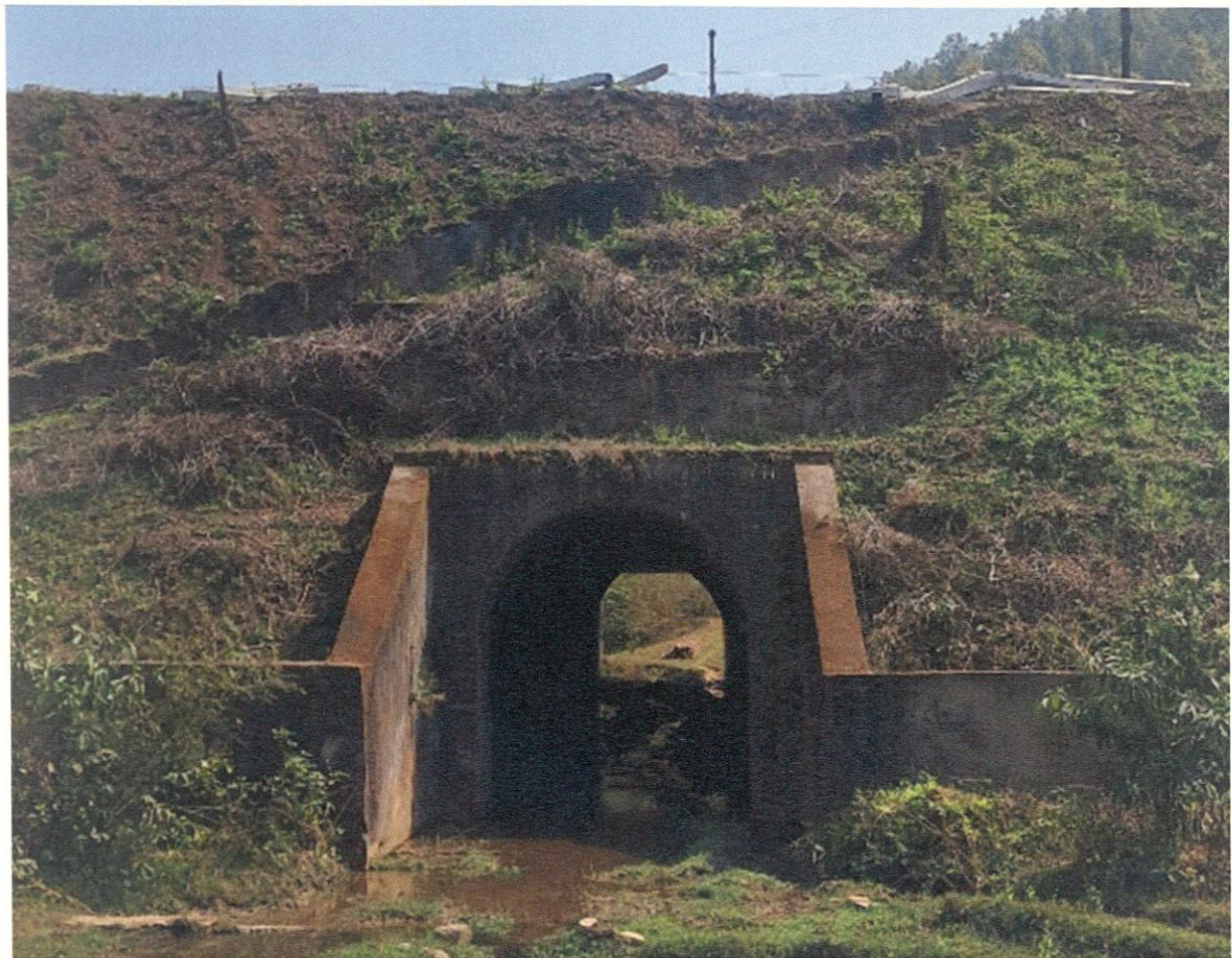
Figure 3.4.6: Existing culverts need structural modifications for elephant underpass
