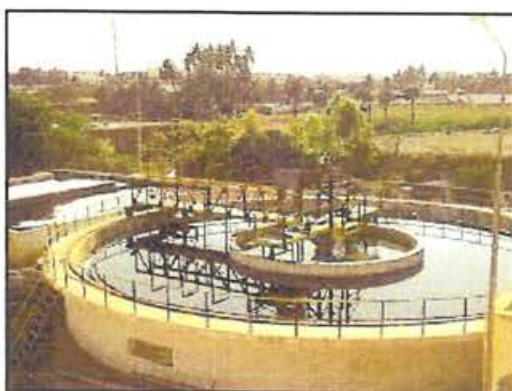
Plate 4.3.2 Clariflocculator unit of the CETP
