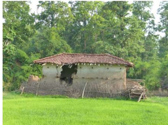
Plate 8.3: A house damaged by elephants in Surajpur district
