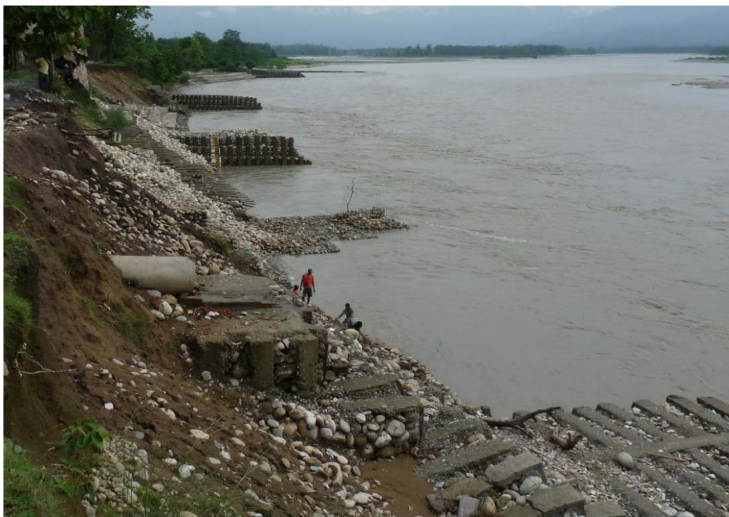
Plate 4.2 Damaged caused to spurs and erosion due to flood in Sharda River
