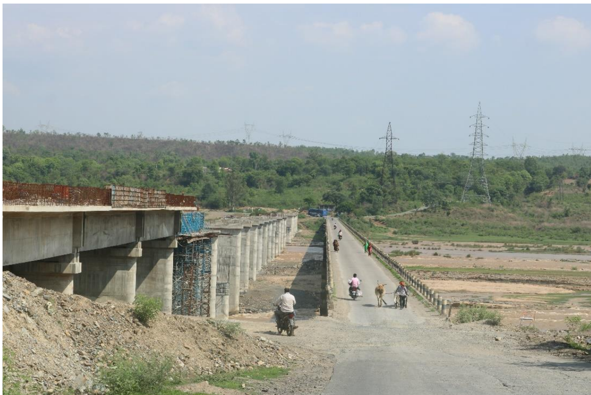
B. Pillars already erected along the river adjacent to the old bridge
