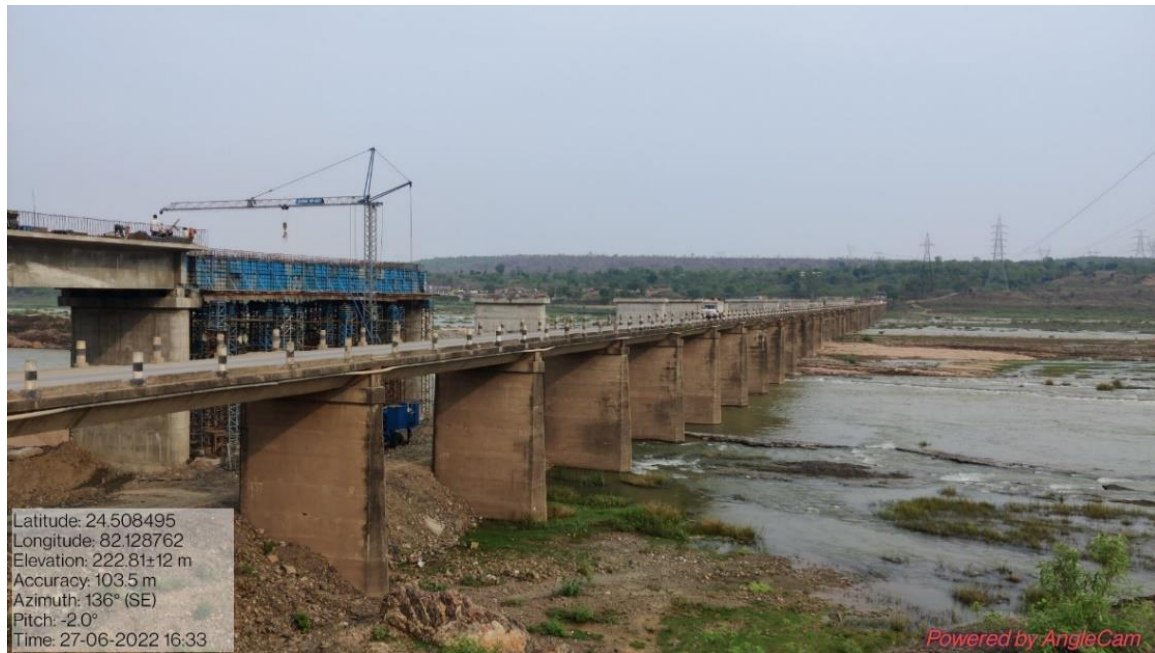
A. Construction work on the new bridge adjacent to the old bridge
