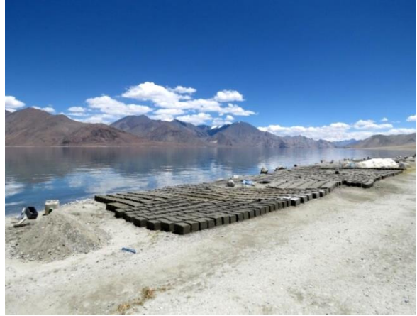
b) Unplanned construction near wetlands
