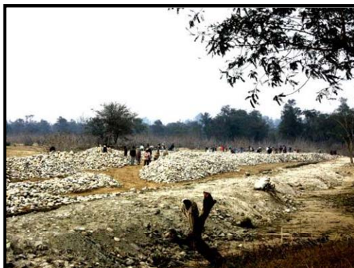
Plate 8.18 Check dam construction at the exit point of drainage from wetland to River Ganga
