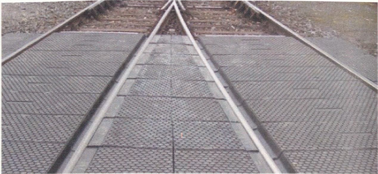
Figure 1. A level crossing with a rubberised surface that can be replicated on level crossings for wildlife.
