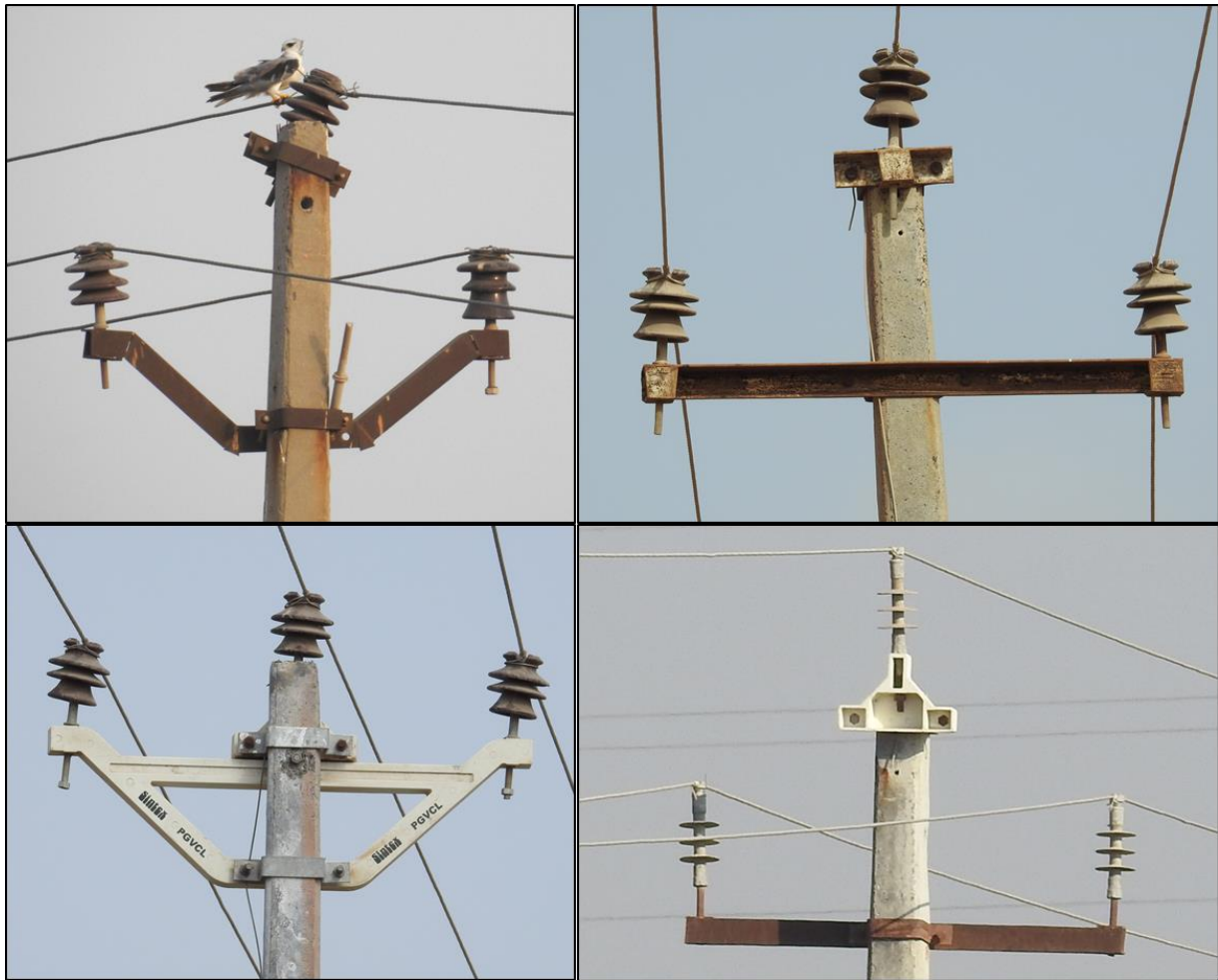
Figure 2. Different types of cross-arms and insulators recorded in the distribution lines in the Kachchh district.
