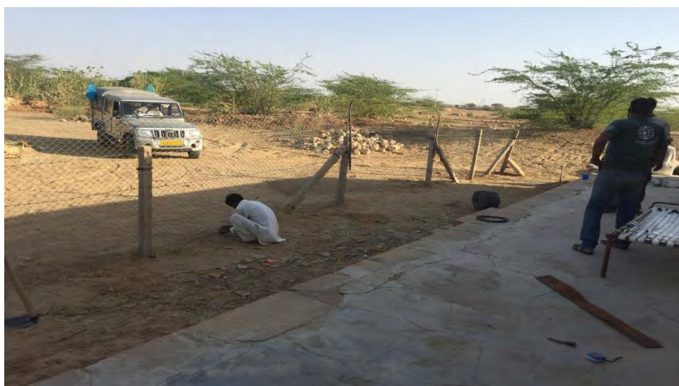
*Fencing around post op facility.
