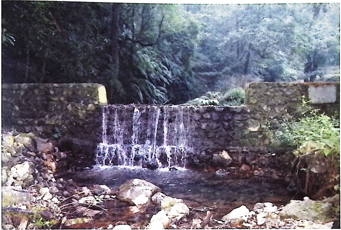
Fig. 13 Check dam structure of Pool M1 showing the concrete wall with wider broad-crested weirs
