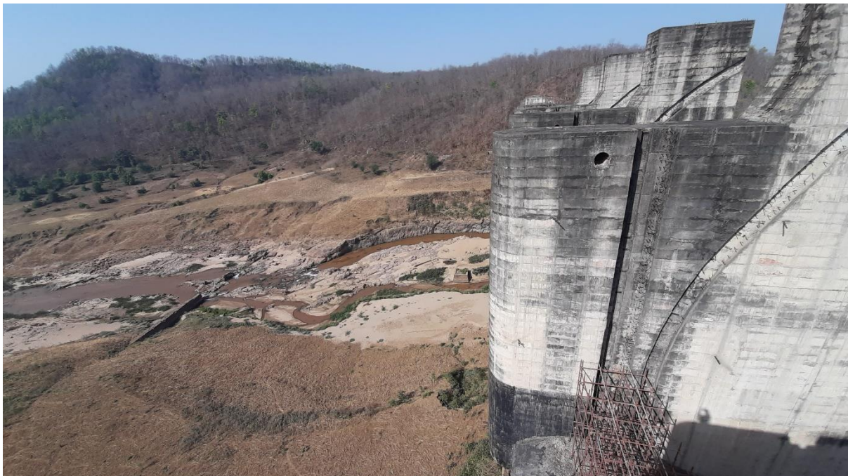
Figure 1: A view of the almost complete Mandal dam on North Koel River near village Kutku, PTR
